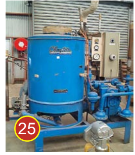
25 Clayton steam boiler.
